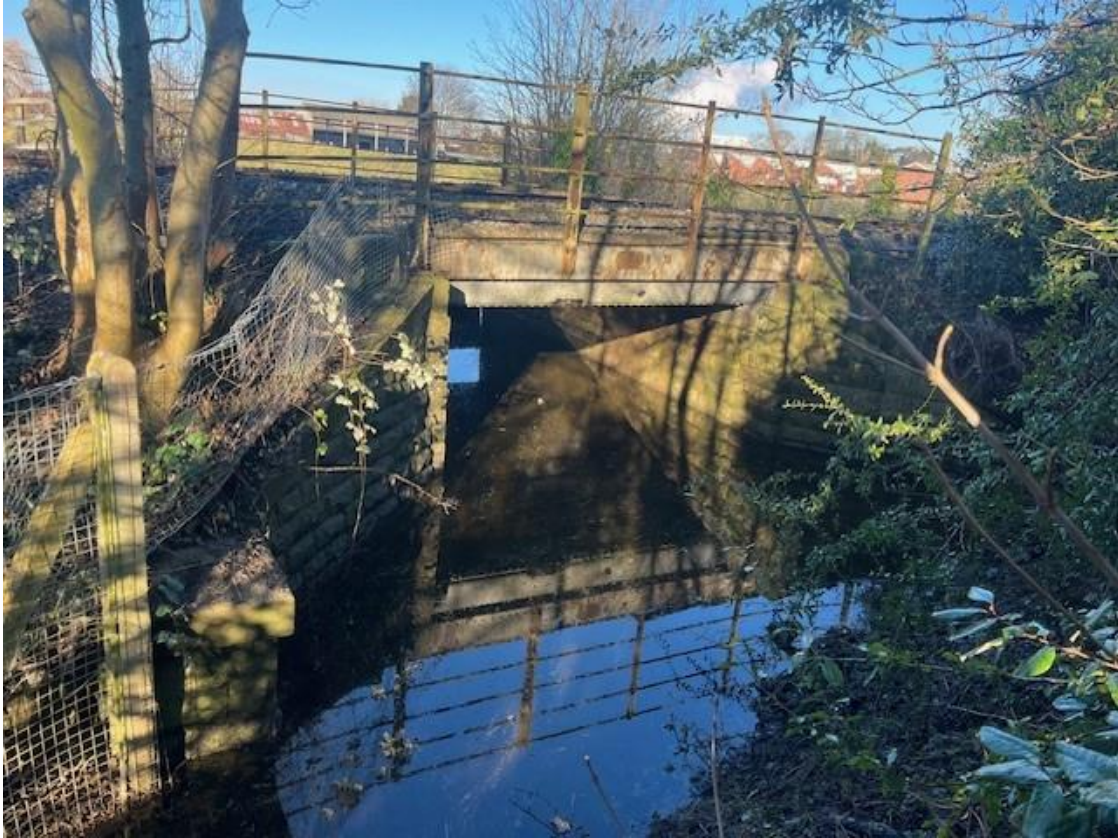
Figure 14: Photo of the existing culvert to east and the associated ditch or trackway. Source: Skanska, 16/01/2025.
